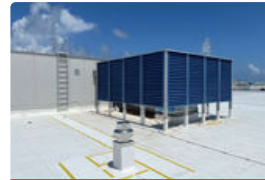
July 2024 Rooftop AC Installed
